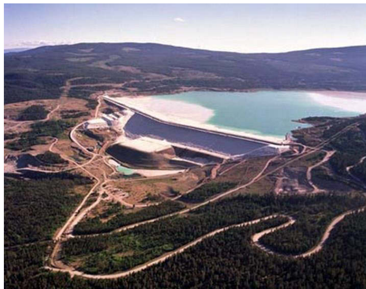
Figure 1 Photograph of a tailings impoundment with part of its boundary formed by natural depression ( http://www.tailings.info/assets/images/content/valleyimpoundment.jpg ).
