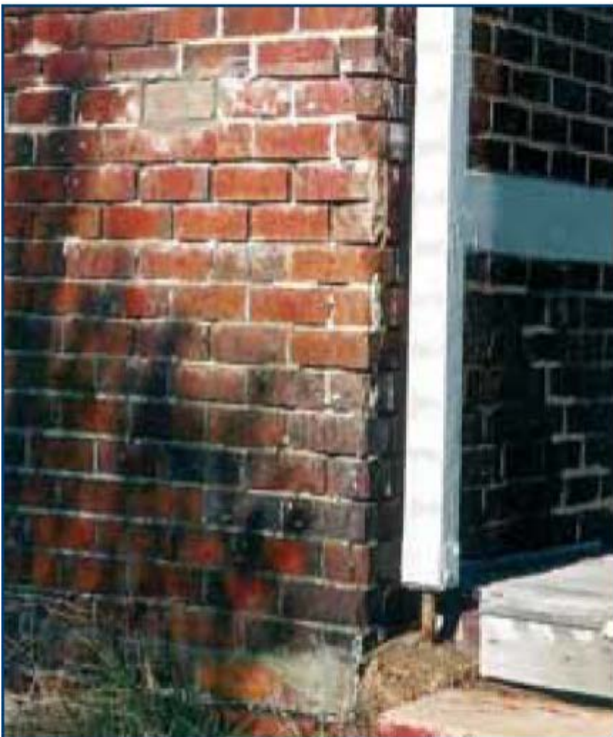
Figure 2.5: Salinity damaged building in rural towns
