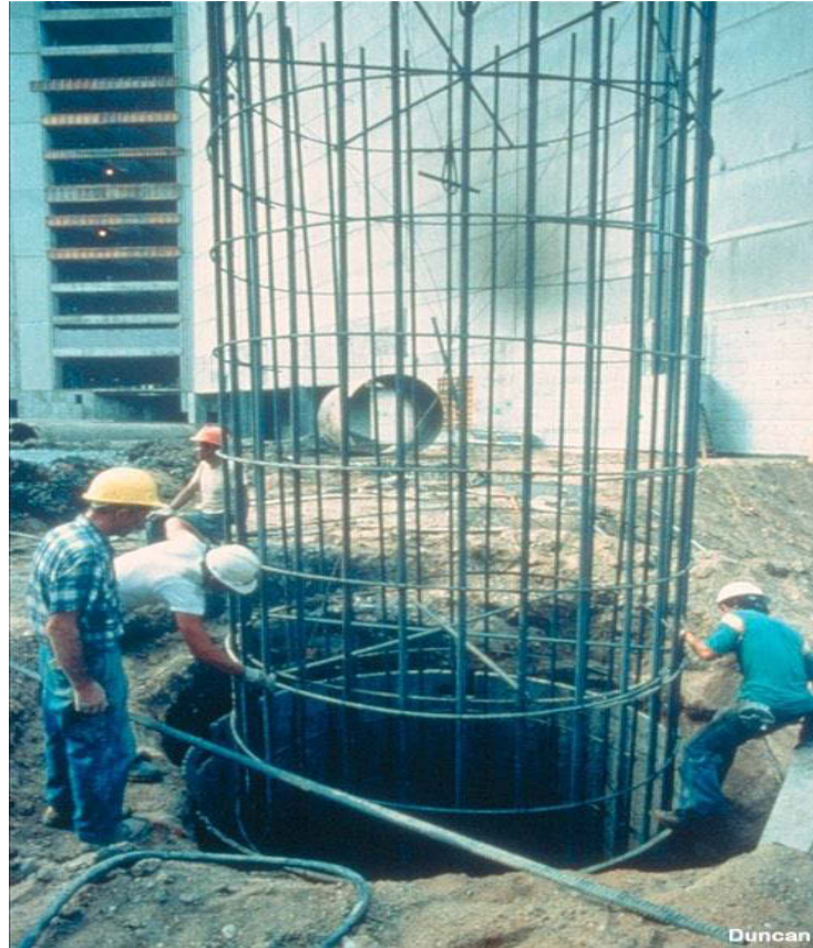
Figure 2-8. A single pile with a case and reinforcements under construction (Photo courtesy of Duncan Priestley Civil Engineering)
