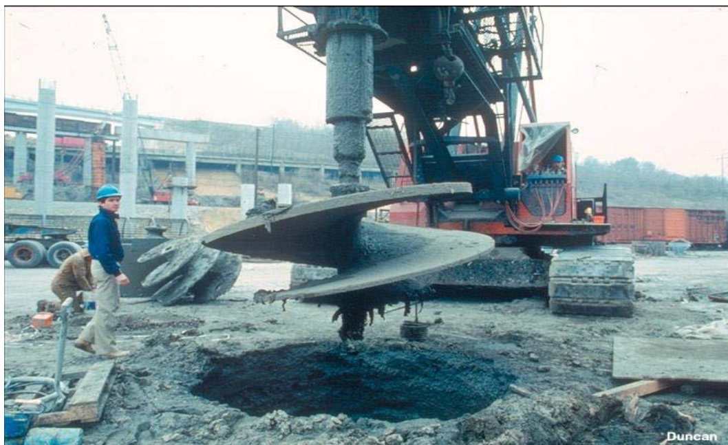
Figure 2-7. An auger used on site for pile installation (Photo courtesy of Duncan Priestley Civil Engineering)
