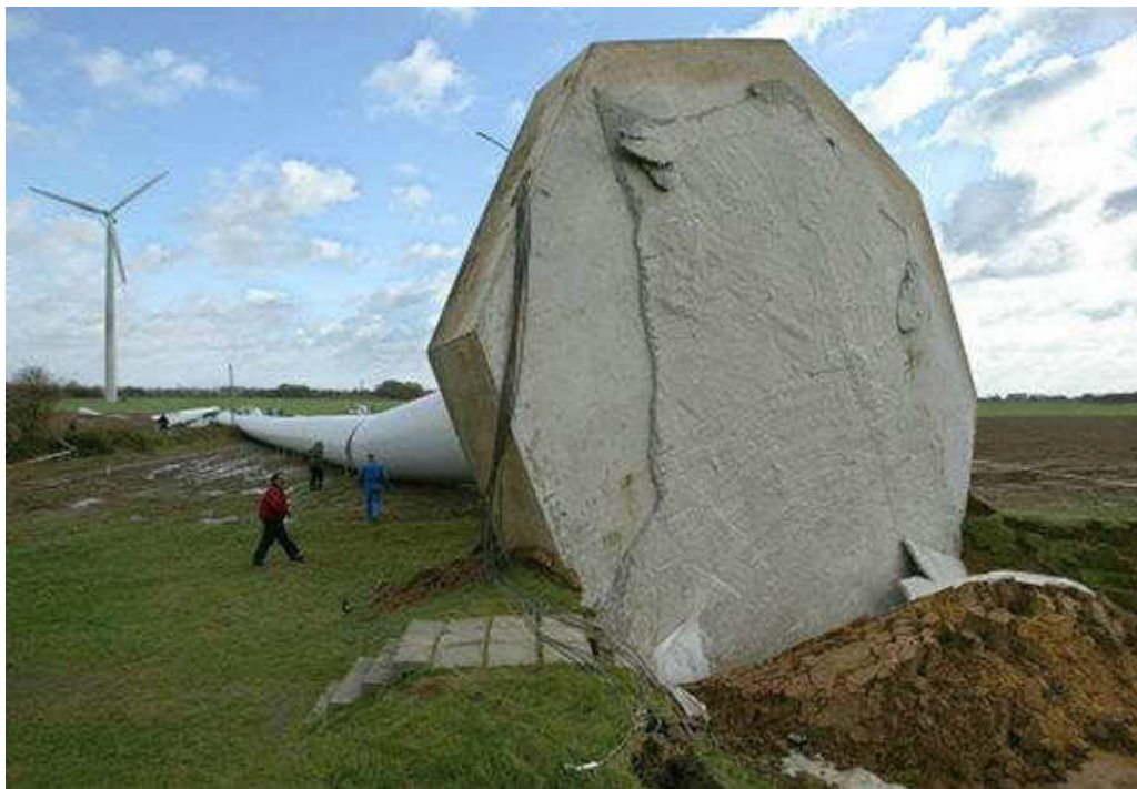
Figure 1-7. Failure of a wind turbine comprising of a tower and a footing (photo courtesy of Con-tech systems Ltd)
