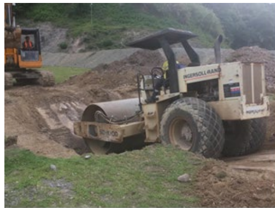
Figure 16. Test locations were backfilled and compacted on completion of block sampling activities.
