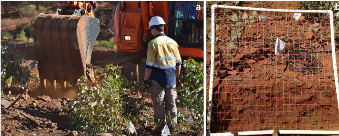
Appendix D a) Using a backhoe to create a soil pit 0.1 m from a plant stem b) sampling pit and frame with 0.0025 m 2 squares used to count the number of roots in each cell on a 0.3 m thick cover.
